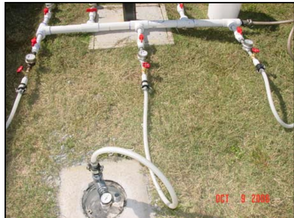
FIGURE 3. Injection manifold and well.
